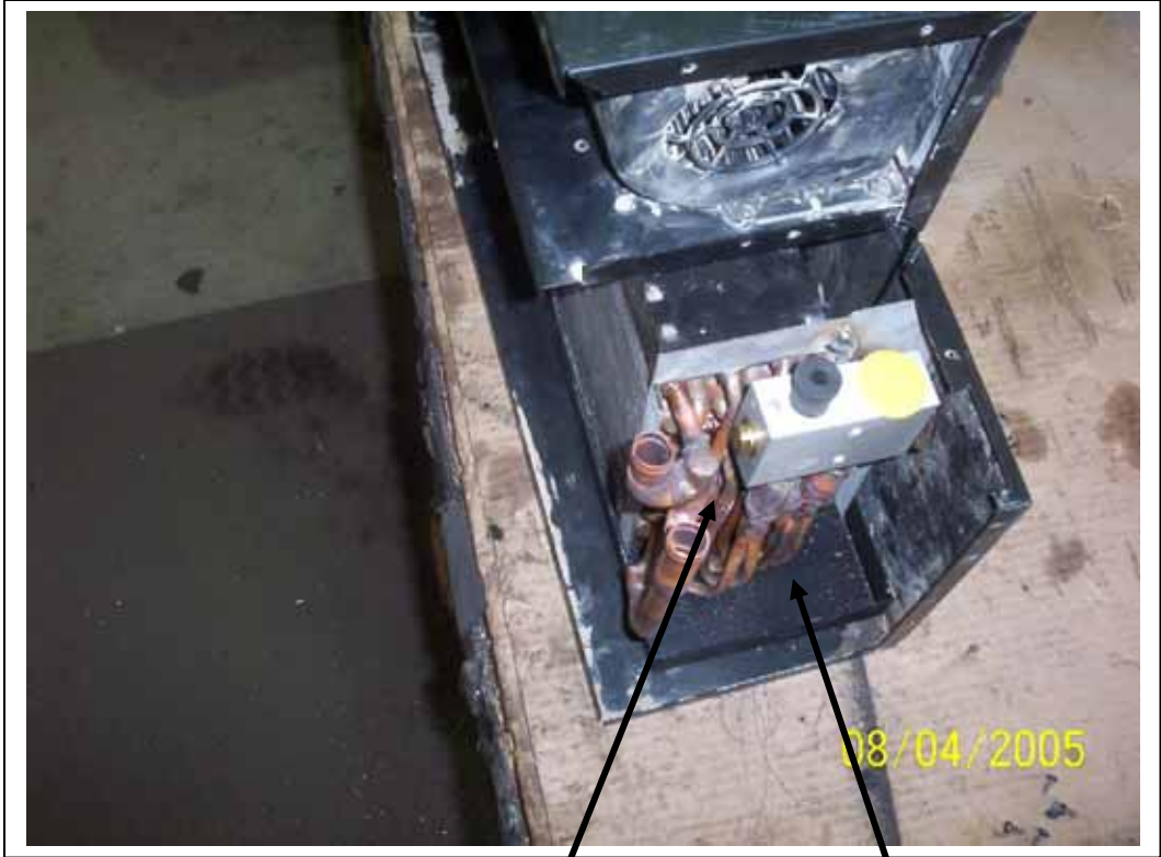
Evaporator/heater coil in place.
