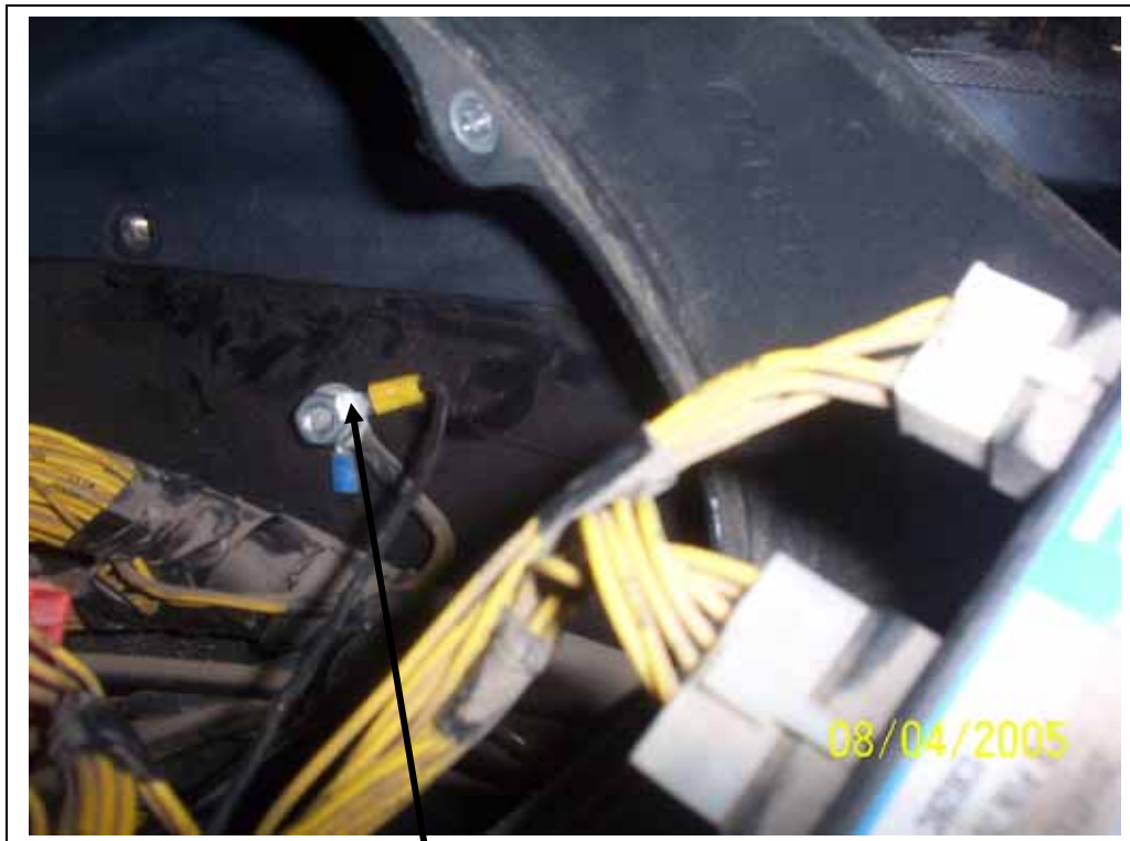
Ground wire from A/C switch.
