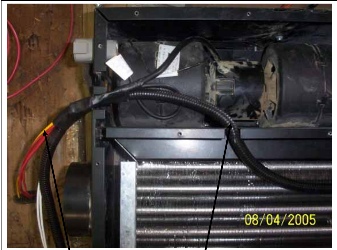
Electrical for power fans with 10" extensions.
